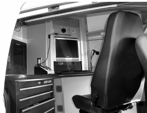
The inside of the van provides a sophisticated computer console and software to capture and store digital images of the sewer pipes.
