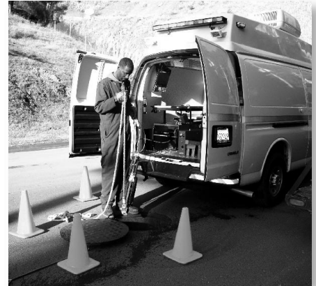
The remote controlled camera is being readied for lowering into the sewer main.
