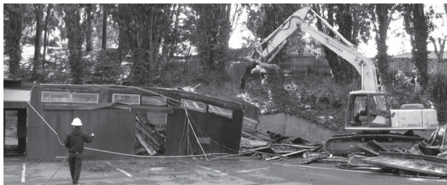
Demolition is almost complete on the site that will house the future Stege headquarters and maintenance yard, which is shown in the upper right drawing.
